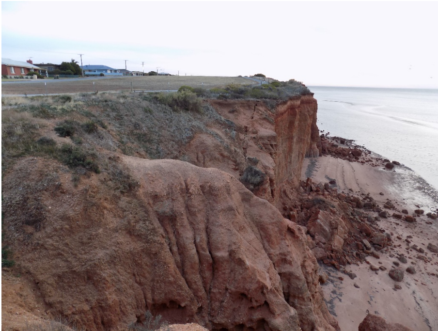
Photo: A recently collapsed part of the cliff line adjacent to the grassland site. The most distant part of the cliff visible in the photo also has a large crack forming a metre or two back from the edge.
