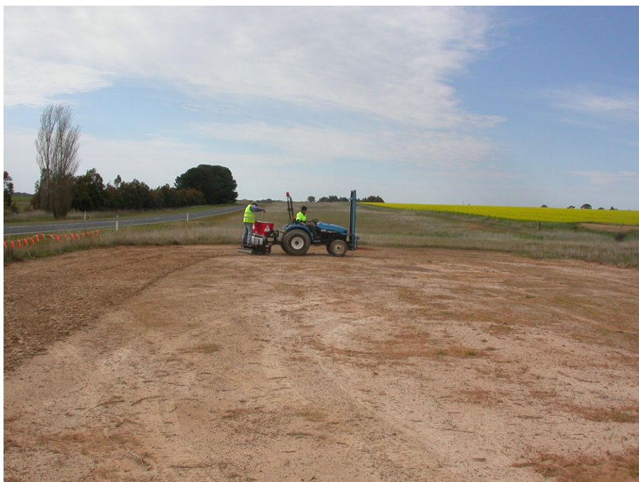
Figure 3. Scalped site at roadside restoration No.1, approximately 3 km west of Wickliffe, Victoria, showing the GGRP seeder in action direct seeding. Scalping is routinely carried out on Greening Australia's grassy reconstruction sites if a site assessment indicates nutrient levels or weeds are likely to be an ongoing problem. (Photo Paul Gibson-Roy).
