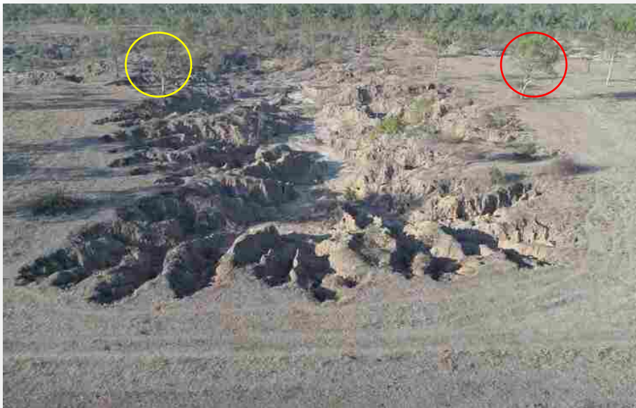
Plate 10 The pre-remediation state of treatment areas 3 (left) and 4 (right) in February 2018. The hay stack contains 415 450kg Rhodes grass hay bales used in the 2018 remediation program.
