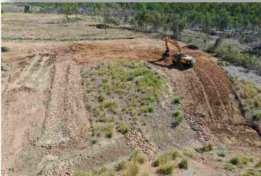
Plate 14 Repairs of the above site underway involving the regarding of the eroded area and construction of a batter chute to take flows (diversion bunds to the throat of the batter chute not yet installed at the time of photo).
