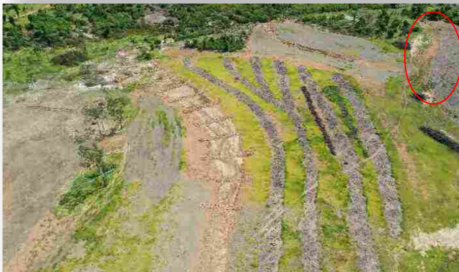
Plate 22 A long low slope batter on the downstream eastern extent of Treatment 8 as a result of a plan redesign necessitated some innovative approaches to slope stabilisation.
