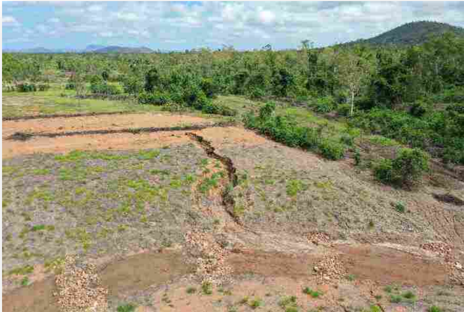
Plate 13 Erosion on the batter face caused by failure of diversion bunds intended to disperse concentrated flow caused by a small drainage depression after earthworks.
