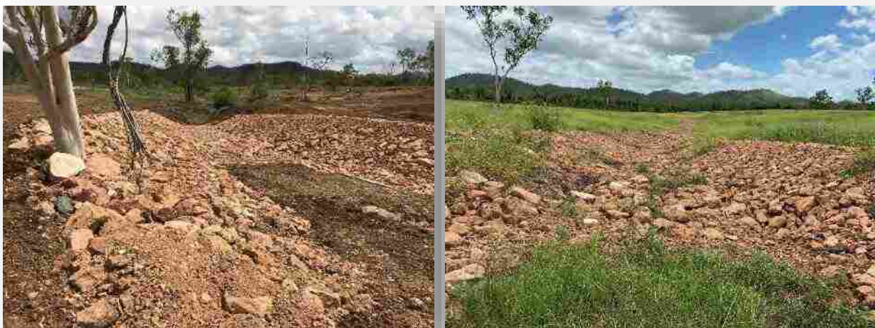
Plate 3 Treatment 5 rock chute installed in November 2017 prior to the Treatment 8 remediation in 2018 (left image), and same site in February 2019 post Treatment 8 and mid 2018-2019 wet season.
