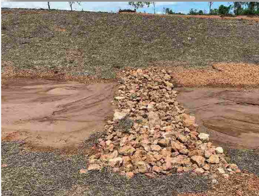
Plate 16 Approximately 200mm depth of sediment deposition behind porous check dams in Treatment 3, flow from photo left to right
