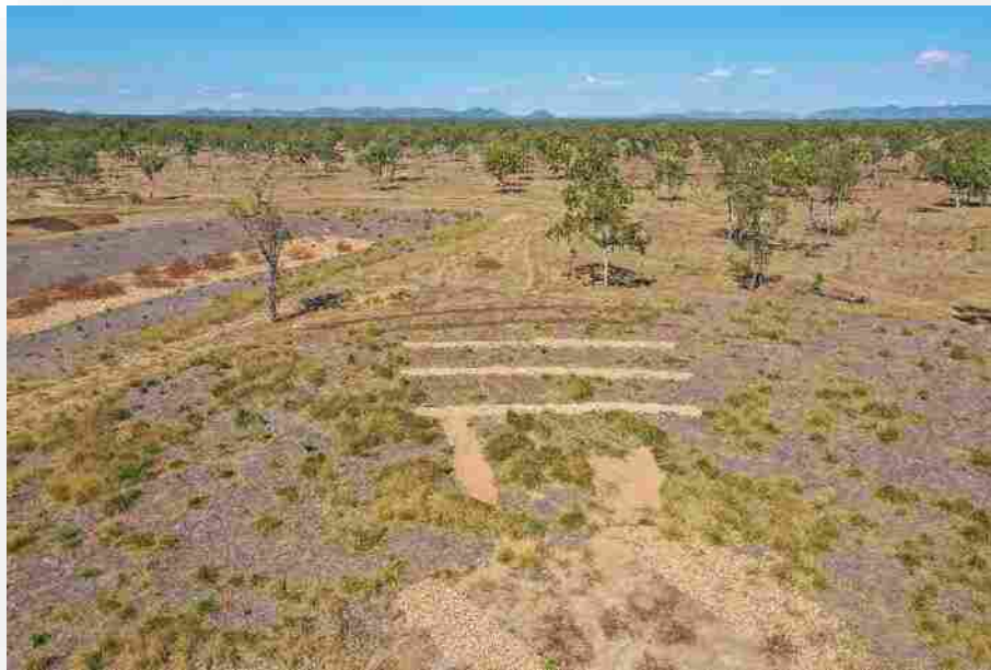
Plate 12 Cobble (50-150mm quarry rock) and bagasse checks installed at the location of rilling on the batter face caused by concentration of overland flow during intense rainfall events.
