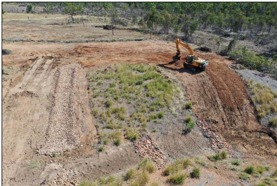
Plate 7 Repairs of the above site underway involving the regarding of the eroded area and construction of a batter chute to take flows (diversion bunds to the throat of the batter chute not yet installed at the time of photo).
