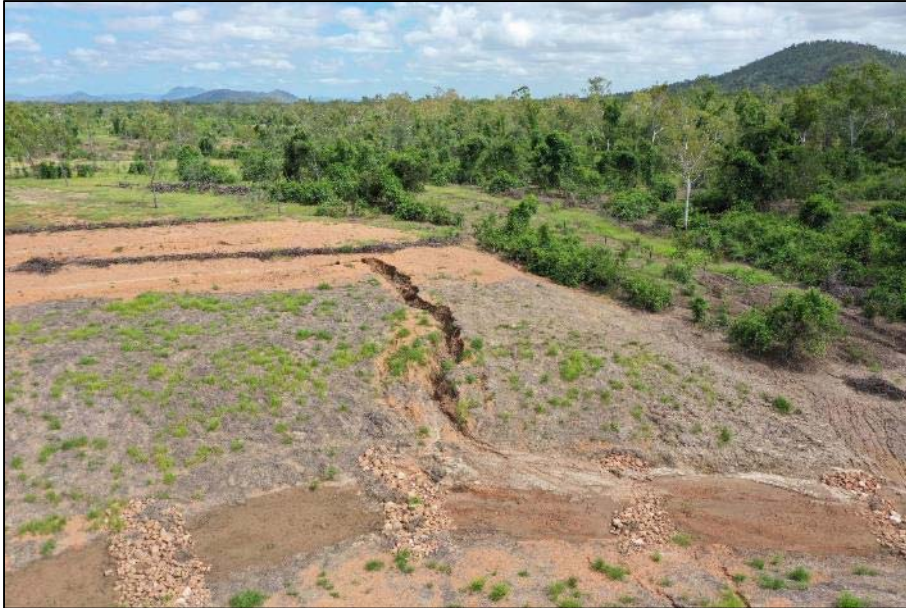
Plate 6 Erosion on the batter face caused by failure of diversion bunds intended to disperse concentrated flow caused by a small drainage depression after earthworks.
