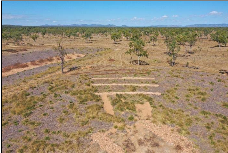
Plate 5 Cobble (50-150mm quarry rock) and bagasse checks installed at the location of rilling on the batter face caused by concentration of flow during intense rainfall events.
