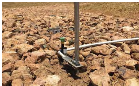
Unidata velocity sensor and ISCO pump intake mounted below with HOBO water level logger (beneath green cap). Photo credit: Fruition Environmental
