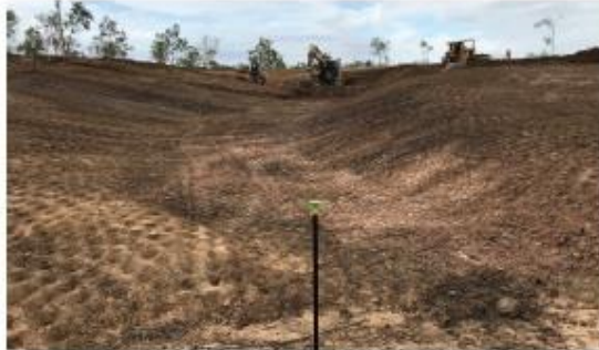
In Treatment 1, regrading the heavily incised gully area to a pre-designed landform was the first task. Care was taken to balance the cut and fill to reduce earthworks costs. Dealing with extensive tunnel erosion was a major challenge on this site.
