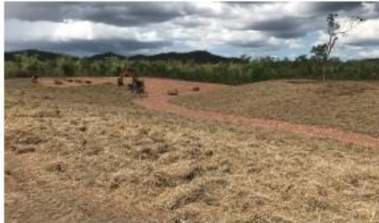
Mulching the batters and all disturbed areas was the second last job on the site. The entire site was re-seeded after rain in March 2018
