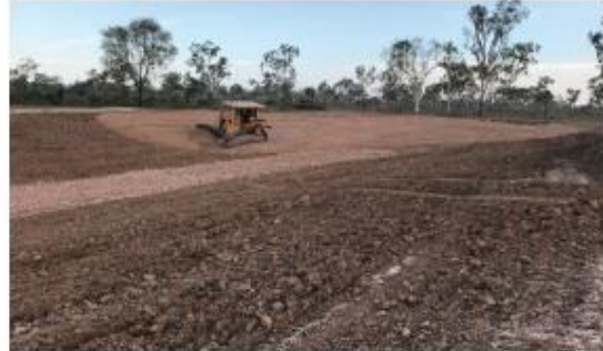
Capping with a 200mm thick layer of rock and soil from the quarry occurred after gypsum was applied (18t per hectare) and ripped into the prepared surface.
