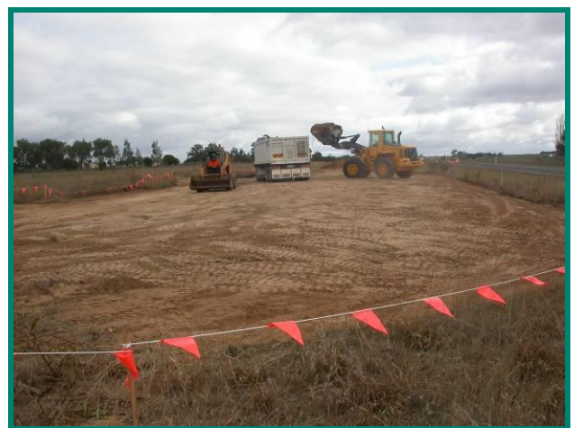
Soil works being undertaken to remove weed loads prior to direct seeding at Wickliffe
