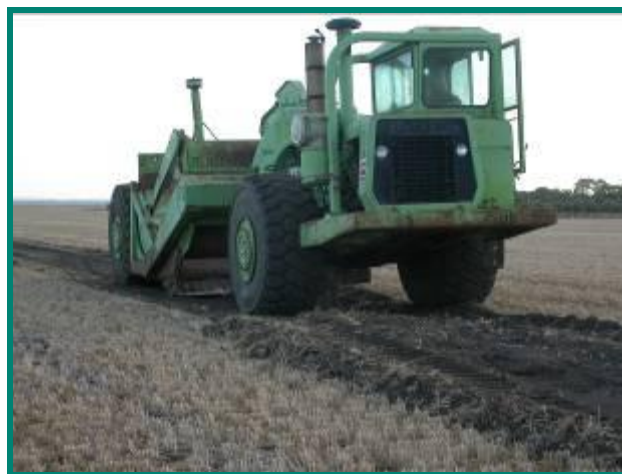
A large "scraper" starting works. In the past we have used bobcats and road graders
